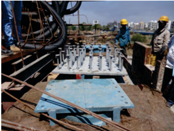
Photo 86 Wrongly installed Pot Bearing
