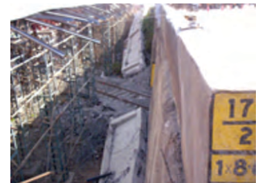
Photo-76 Girder toppled down
