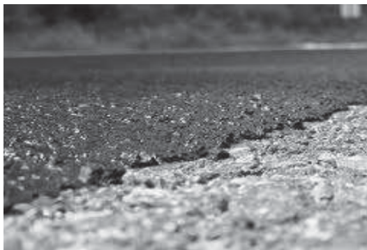
Photo 3.1 Terasurfacing on Distressed bituminous surface
