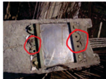
Photo-75 Missing Anchor Sleeve
