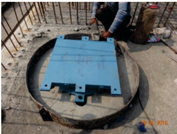
Photo 88 Wrongly installed Pot Bearing
