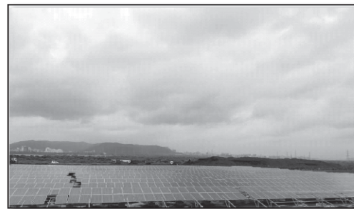
Solar on Grid Installations
