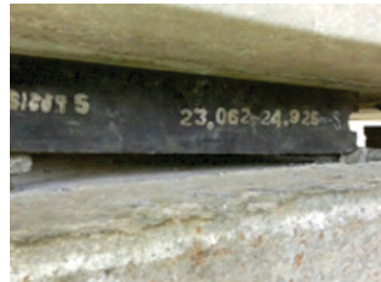
Photo-70 Pedestal is not horizontal
