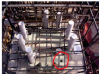
Photo-74 Missing Anchor Sleeve
