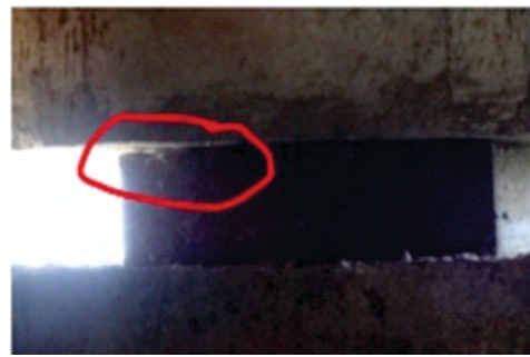
Photo- 68 Gap at top of Bearing
