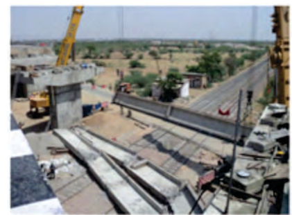
Photo- 79 Girder toppled
