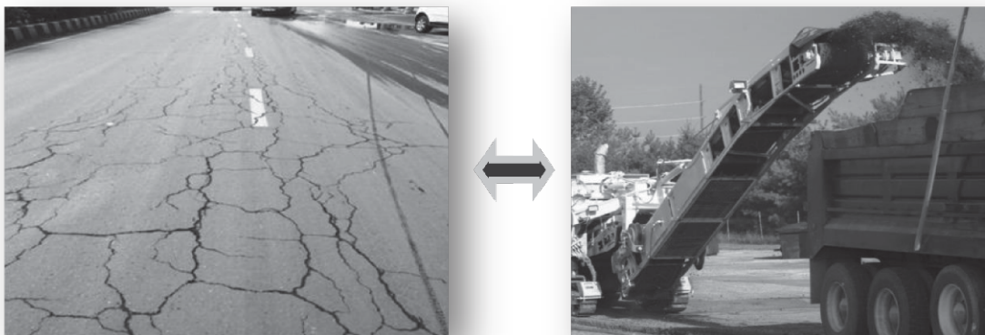
Photo 2.1 Distressed Bituminous surface Milled through Milling Machine for Extraction of RAP
