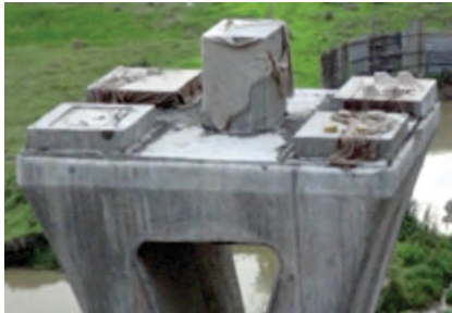
Photo-90, Sismic Block on Pier Cap
